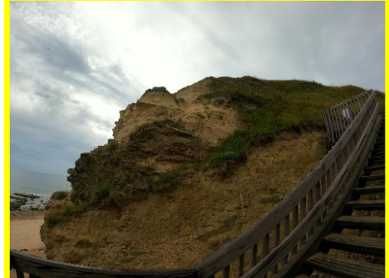
Cracking through the rock overhang adjacent to structure (/0401C01)
