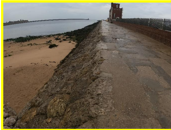
South Pier in overall fair condition along northern face, landward end (/0103C01)
