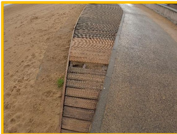
Damaged timber boardwalk near the Sand Dancer public house (/0201C03)
