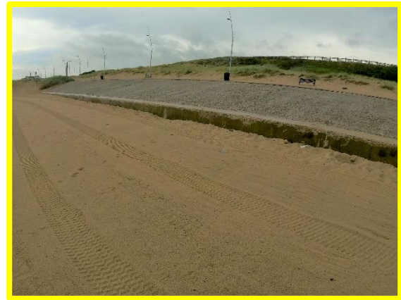
Cracking to render on wall at rear of promenade (/0202C06)
