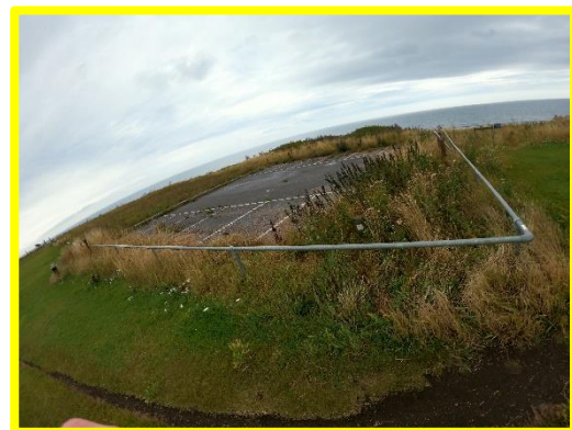
Closed car park due to large cliff failure (/0402C01)
