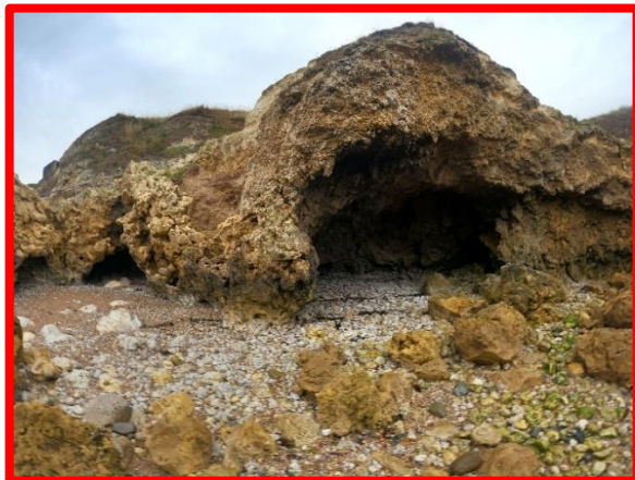
Two large caves undermining access point adjacent to Camel Island (/0401C04)
