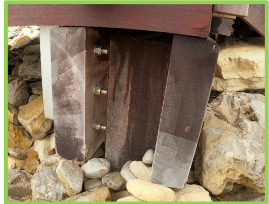
Minor damage to structural timbers (/0401C01)
