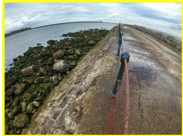
Heavily corroded section of handrail seaward of the access gate (/0103C01)
