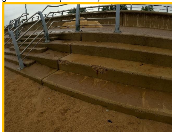
Damaged stepped edge exposing reinforcement (/0102C04)
